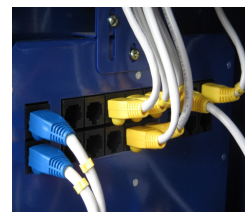
Modular structured cable management design for efficient and clean look that provides ease of maintenance.
